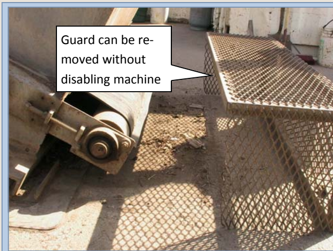
No measures taken to prevent guard removal.
